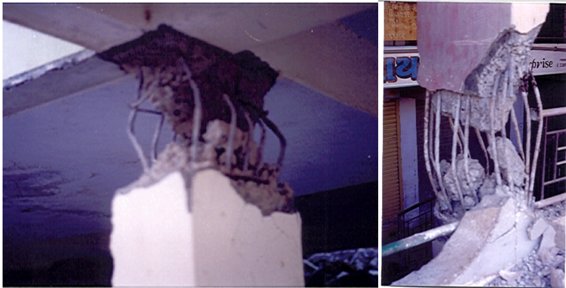
Figure 24: image showing damage in columns due to dynamic loading (credit: TESRA ppt)
