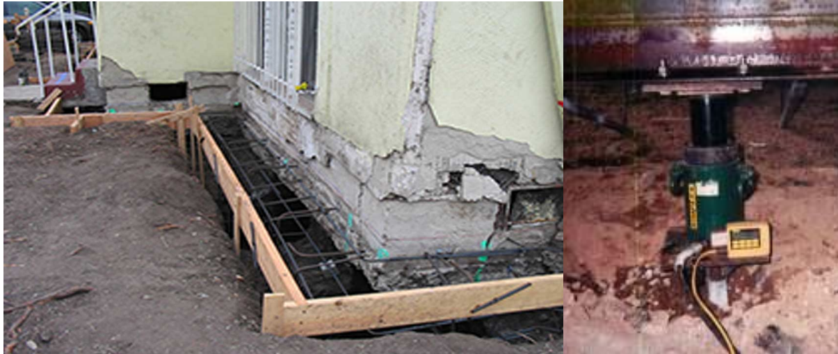
Figure 16: Image showing example of Retrofitting foundation using Jacks and extra reinforcement (credit: www.renotahoe.foundationrepair.com )
