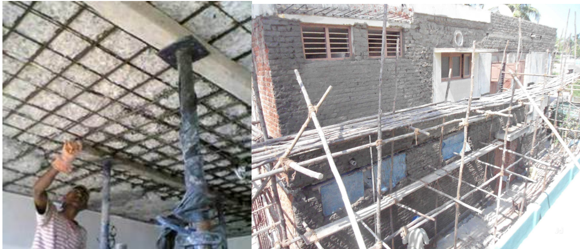
Figure 12: Image showing re-plastering and restoration of slab (left), Restoration process of front facade of building (right). (credit: RMS civil repair works)
