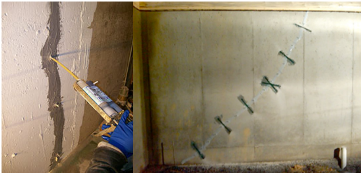
Figure 11: Image showing repair of crack using injection technique (left), repair of crack using diagonal bracing (right). (credit: www.a1crackrepair.com )
