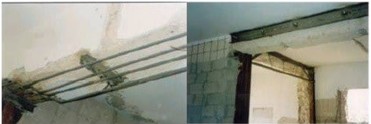
Figure 33: jacketing by bars in beam (left) and Strengthening by steel plate (right) (credit: researchgate)
