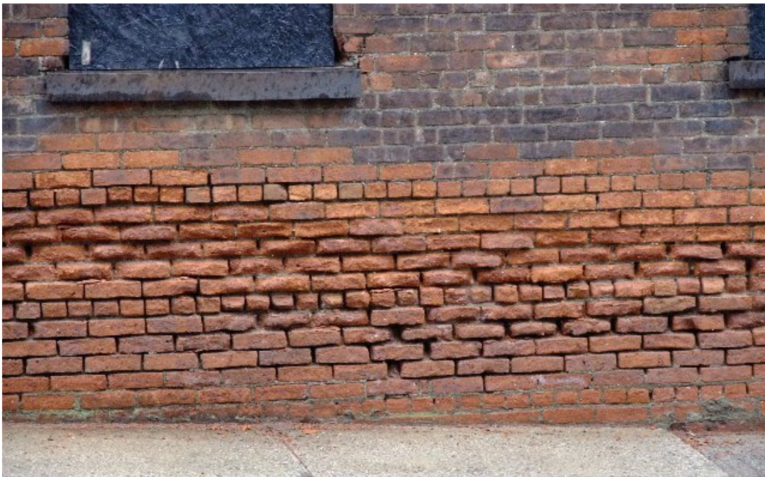
Figure 42: Image showing erosion of mortar due to flood water (credit: inspectapedia.com)
