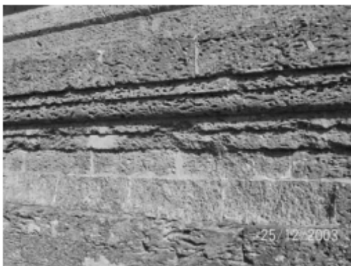
(a) Granular disintegration
