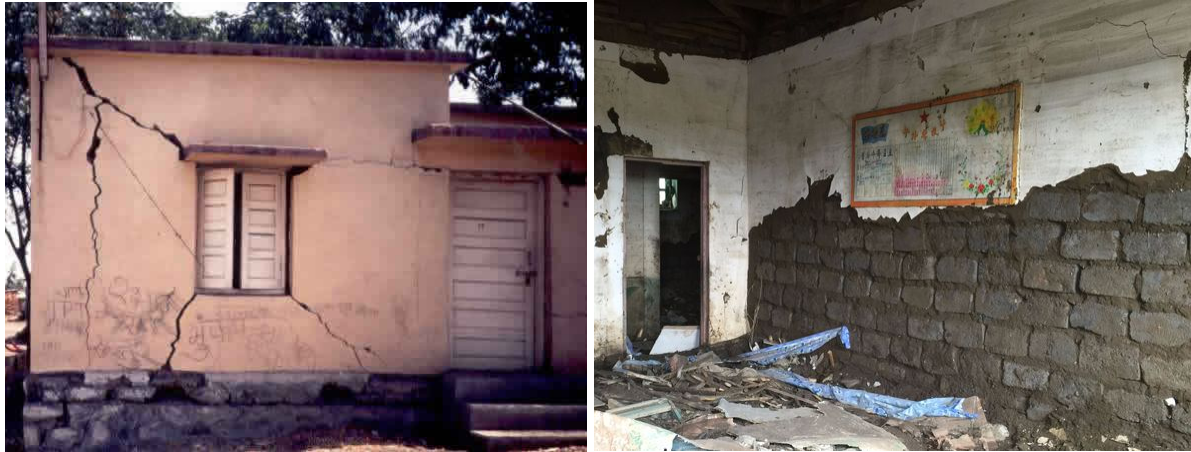
Figure 37: structural damage around opening (left) and damage due to flood (credit: http://db.world-housing.net )
