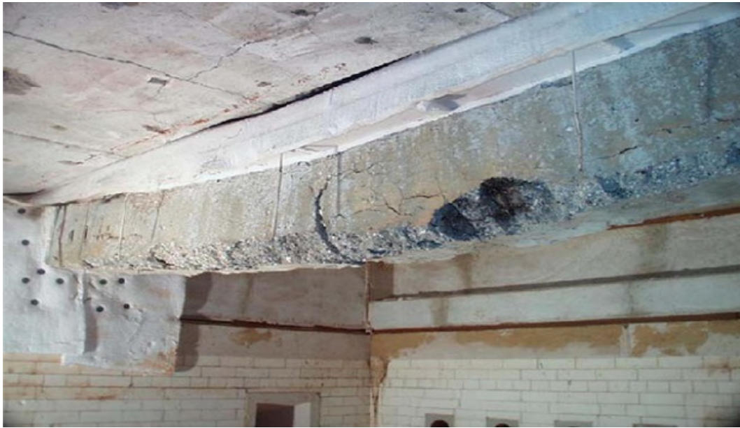
Figure 28: damage due to sagging (credit: daily civil)
