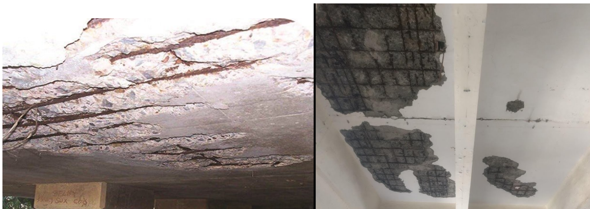
Figure 34: de-lamination and rusting in slab (left) and de-lamination of plaster in slab (right) (credit: researchgate)
