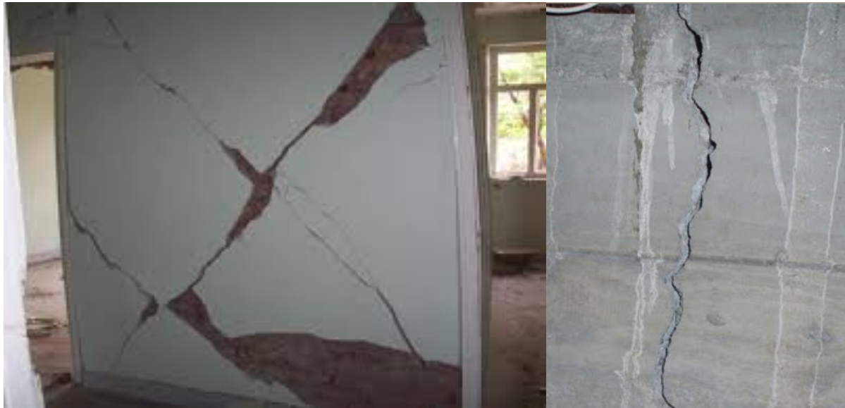
Figure 18: Image showing example of structural cracks in wall due to flood (credit: www.iitk.ac.in )
