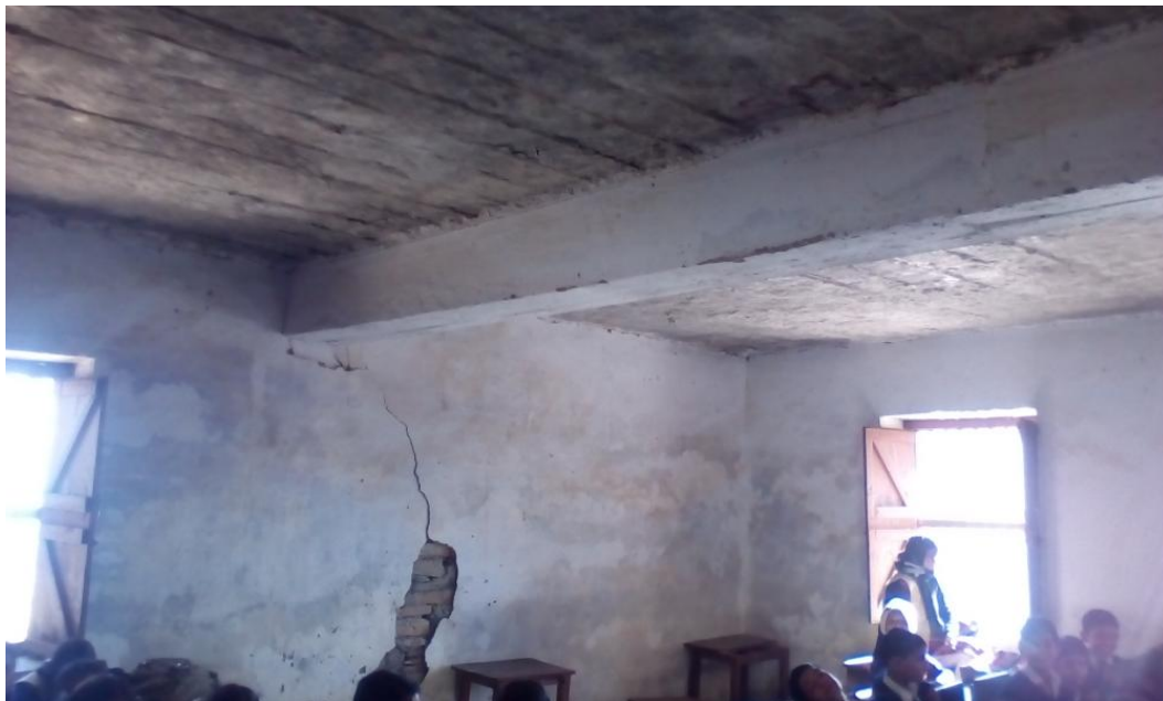
Figure 29: damage in wall and slab due to sagging (credit: daily civil)
