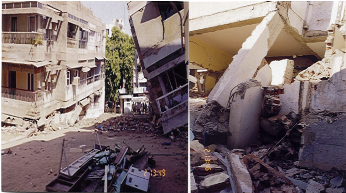
Figure 25: Collapse pattern due to soft story failure due to column failure (credit: TESRA ppt)
