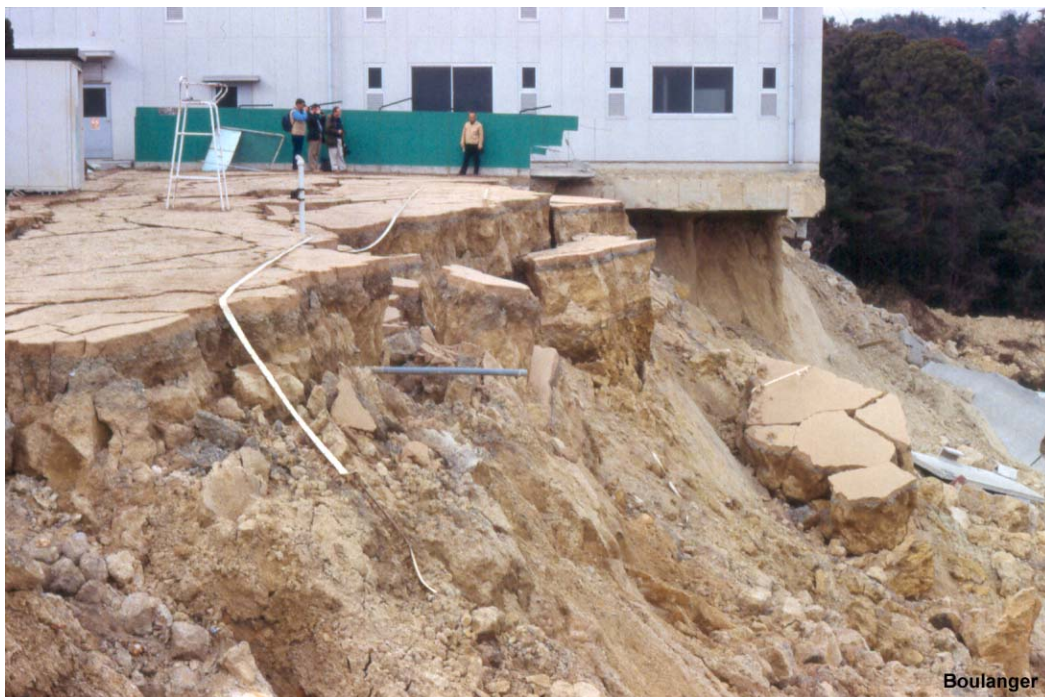
Figure 46: Base soil under foundation eroded due to landslide (credit: http://www.stuff.co.nz )
