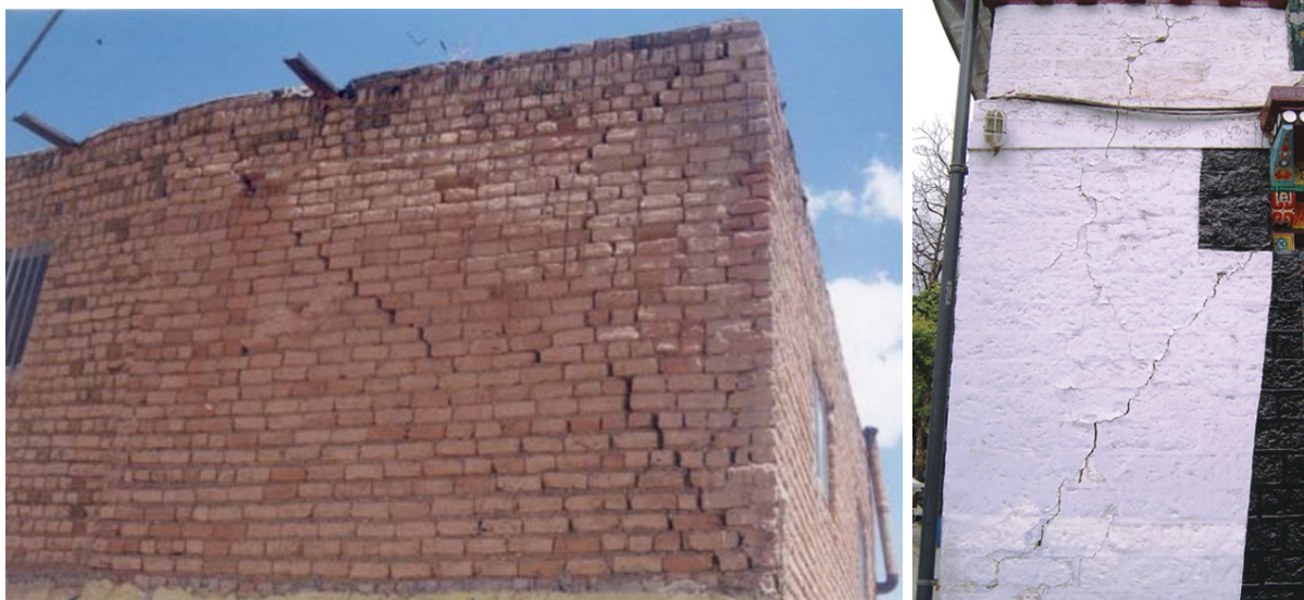
Figure 19: Image showing example of structural cracks in wall due to landslides (credit: ascelibrary.org )
