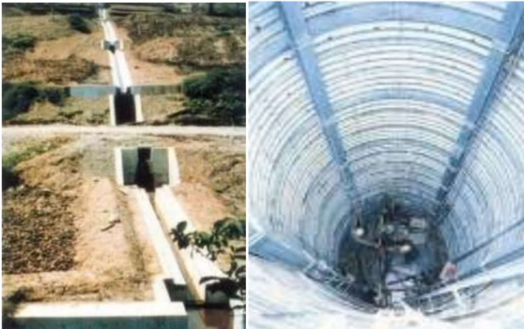
Figure 19: surface drainage ditches (left) and wells for ground water drainages (right) (credit: popescu & sasahara 2010)
