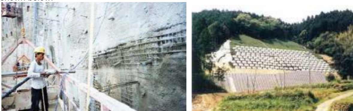
Figure 20: Soil nailing (left) and soil anchoring for slope stabilization (right) (credit: http://www.stuff.co.nz )
