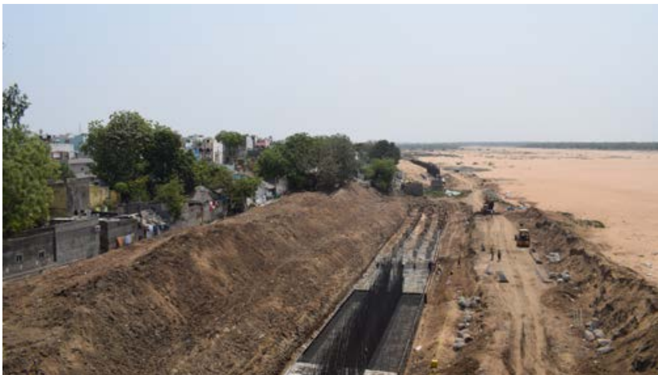
Retaining wall under construction in the floodplains of River Krishna in Vijayawada 37
