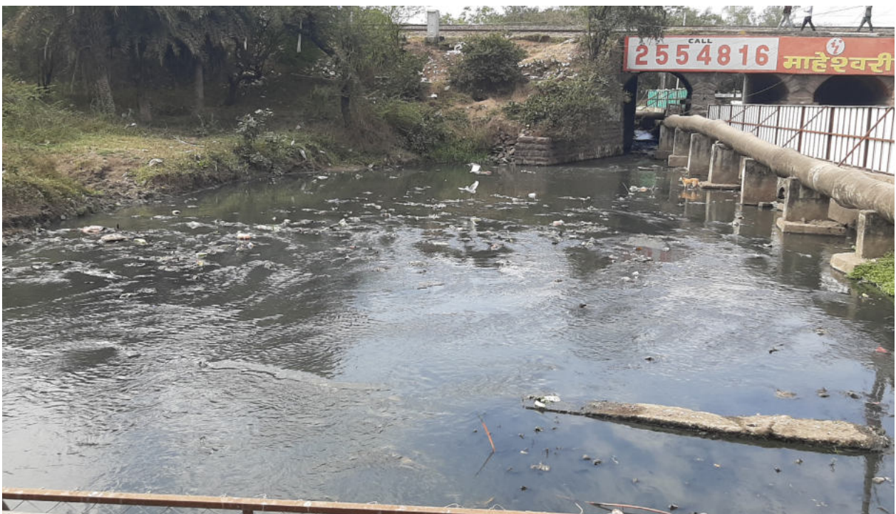
Image 4.9: Flow of sewage into storm water drain near ISBT, Habibganj
